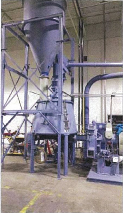
View of the installation at the facility.
