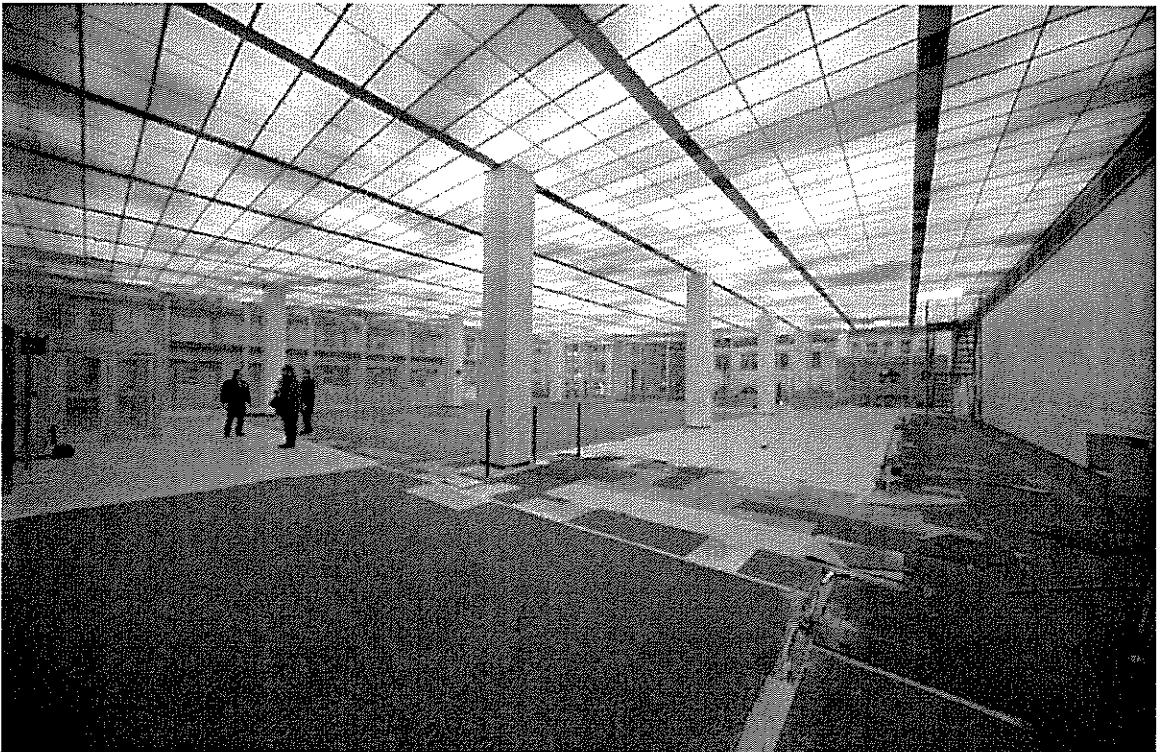
Second floor View east toward Fifth Avenue (upper); view northeast (lower) Photo: Christopher D. Brazee, 2011
