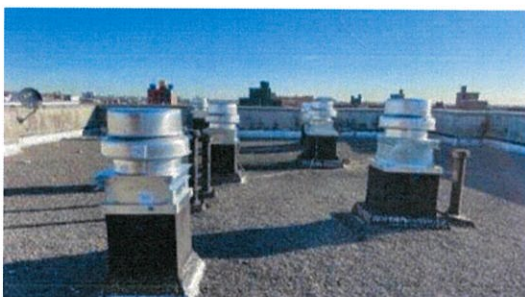
New roof fans
