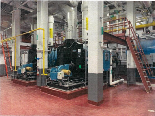
New boilers at Cypress Hills
