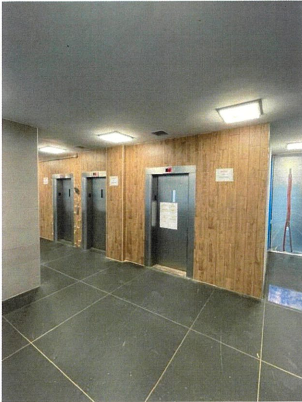
New elevators at 344 East 28 th Street
