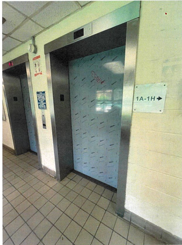
New elevators at Union Avenue Consolidated
