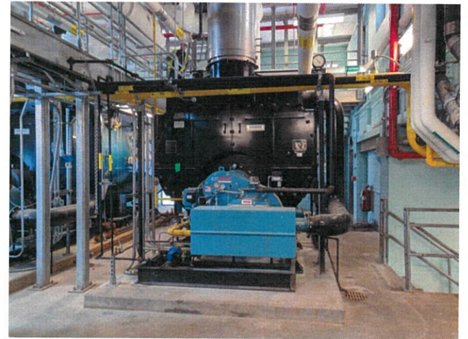
New boilers at Coney Island Houses
