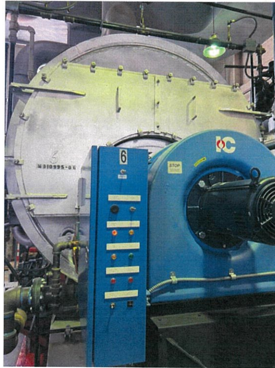
New boiler at Boulevard Houses (PACT)
