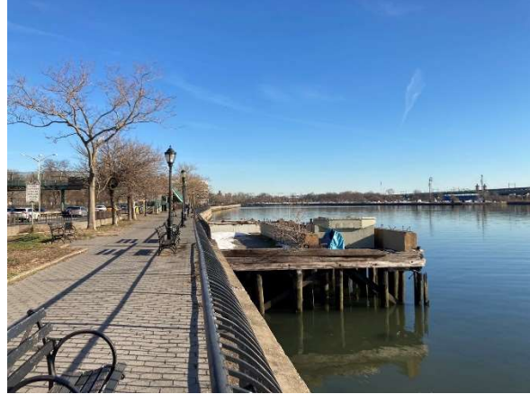
Photo 5: The smaller pier at 110 th street is deteriorated and closed to public. It could be destination for fishing or sitting, away from FDR.
