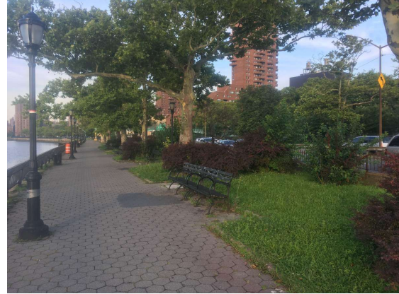
For comparison and to show potential: Around 112 th street across from Thomas Jefferson Park, this brief section has better planting and not yet any collapsing sink holes. In addition to repairs needed elsewhere, preventative structural work will be needed to preserve the remaining places like this.
