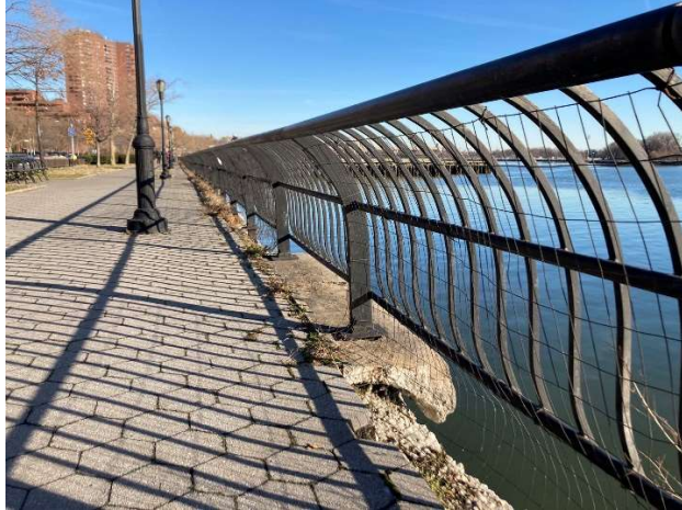
Photo 3: Typical Railing near 105 th Street looking north. Concrete is deteriorating under the rails. Balusters in background are not attached to anything as the concrete is missing
