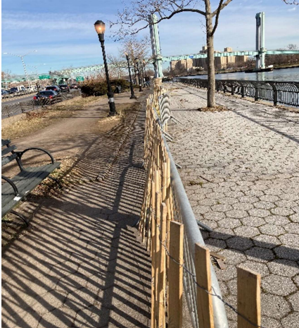
Fencing around multiple sinkholes often leaves only a narrow strip of bare earth between fencing and the FDR
