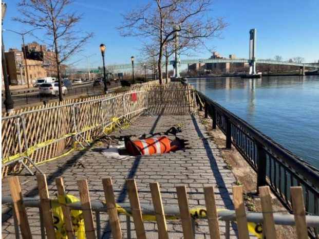
Photo 2 Looking north from 98 th St. Another sinkhole from tidal action. The FDR drive can be seen to left, adjacent to eroding structure.
