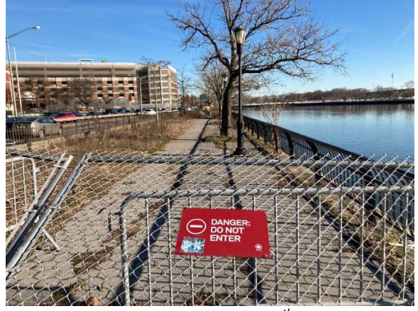
Photo 7: Esplanade north of 114 th street has all been closed for safety concerns from structure. See "D" on Keymap, page .
