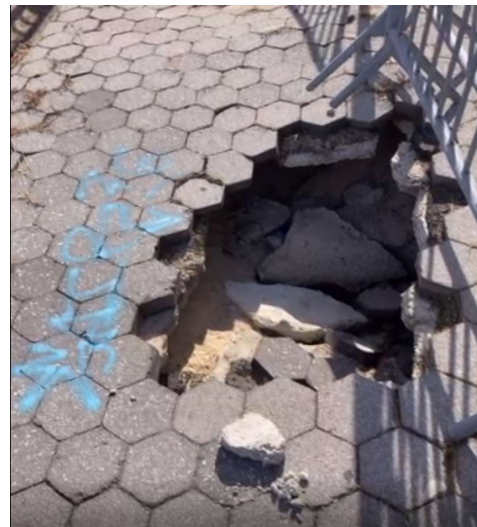
Close up of the same sink hole. See "A" on the keymap, page 3.
