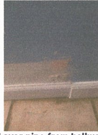
cocked over pipe from hallway radiator February 3, 2016 at 2:35:36 PM
