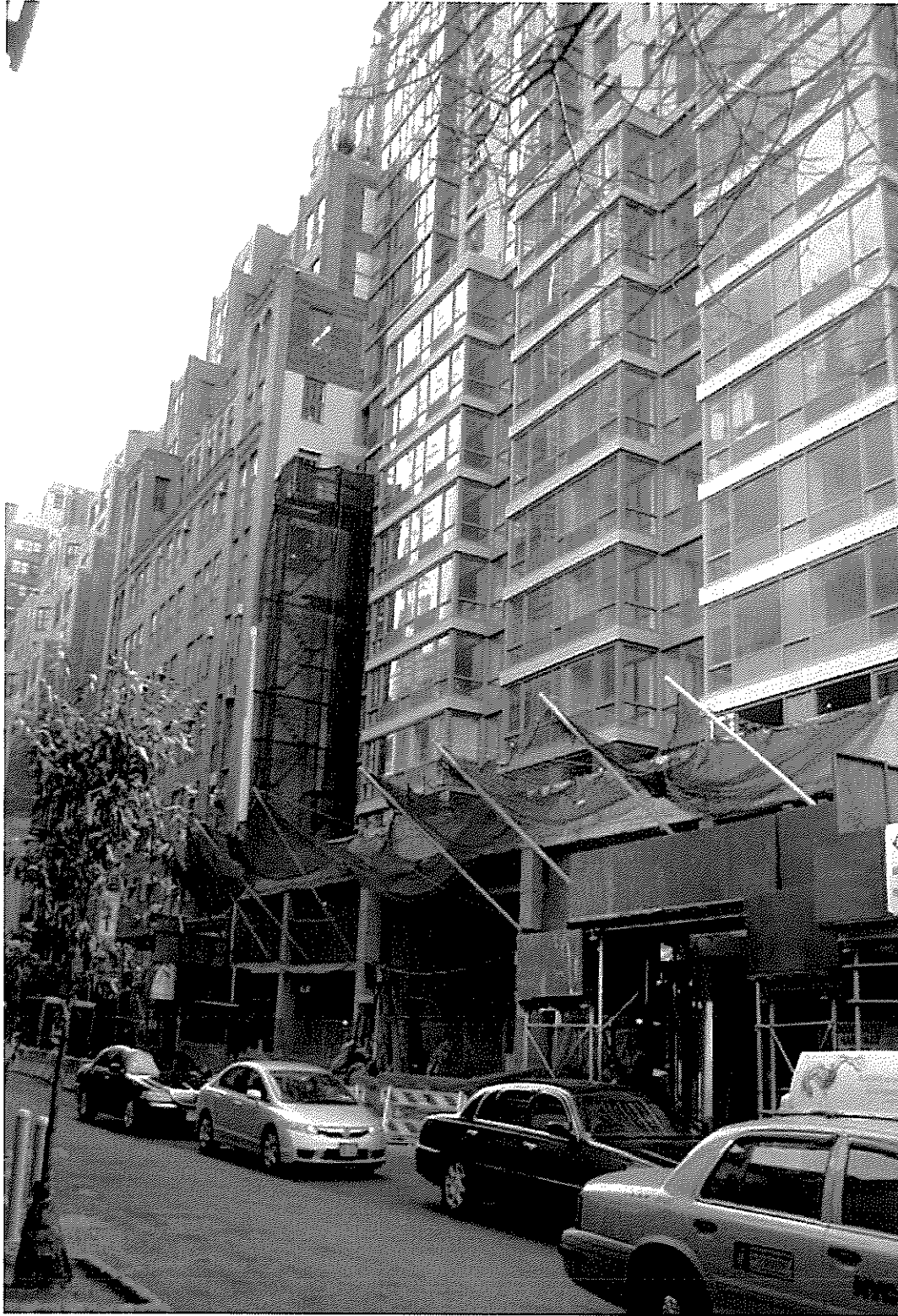
Building not providing street wall that matches existing context
