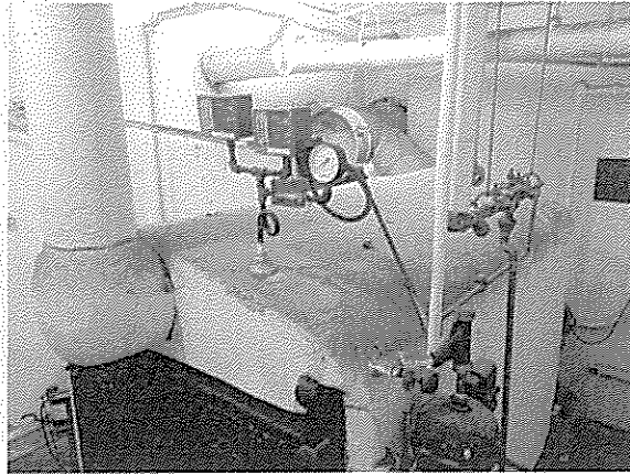
Queens Village HVAC
