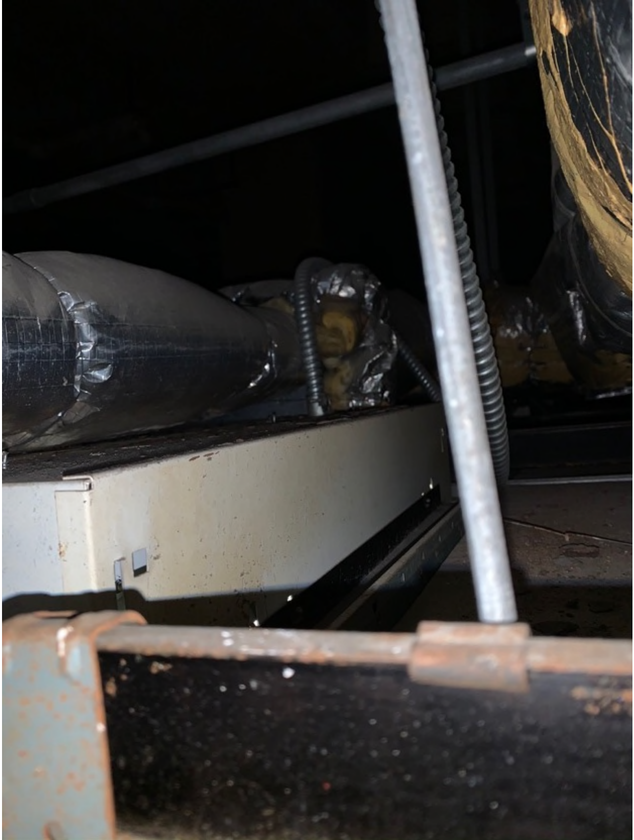
Above the ceiling the slot on the light fixture is open to a return plenum"
