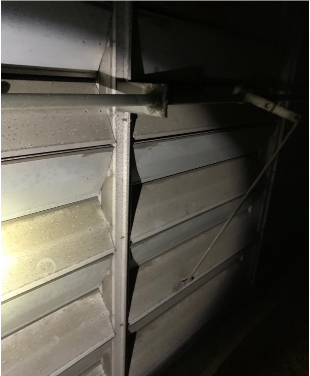
Outside air damper closed on air handler
