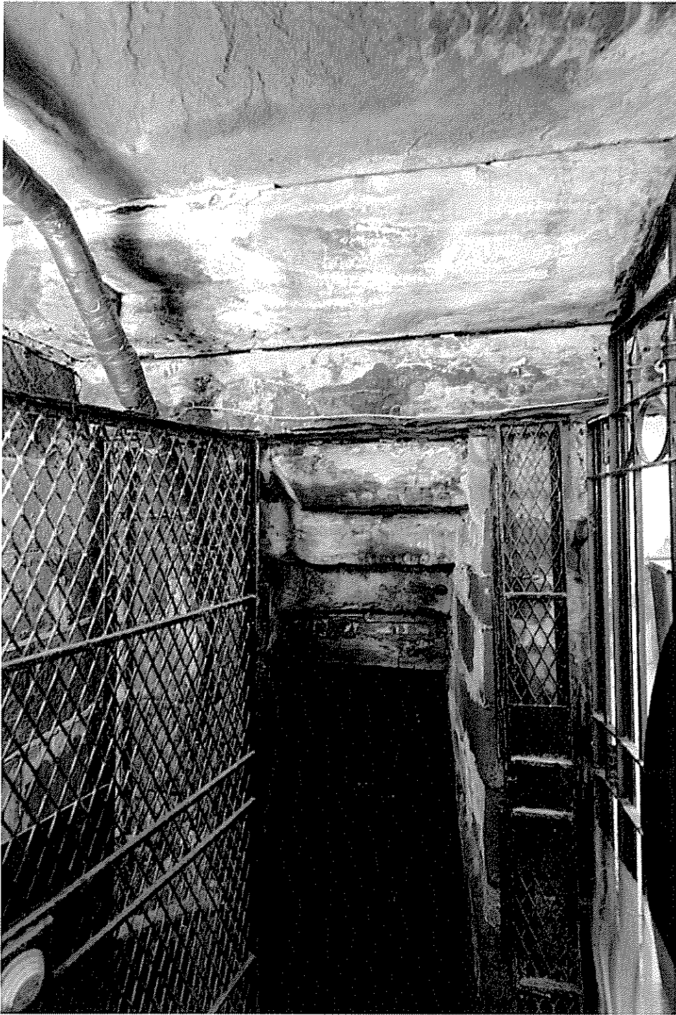
34 Dominick Street LP 2481 Evidence of buried stoop
