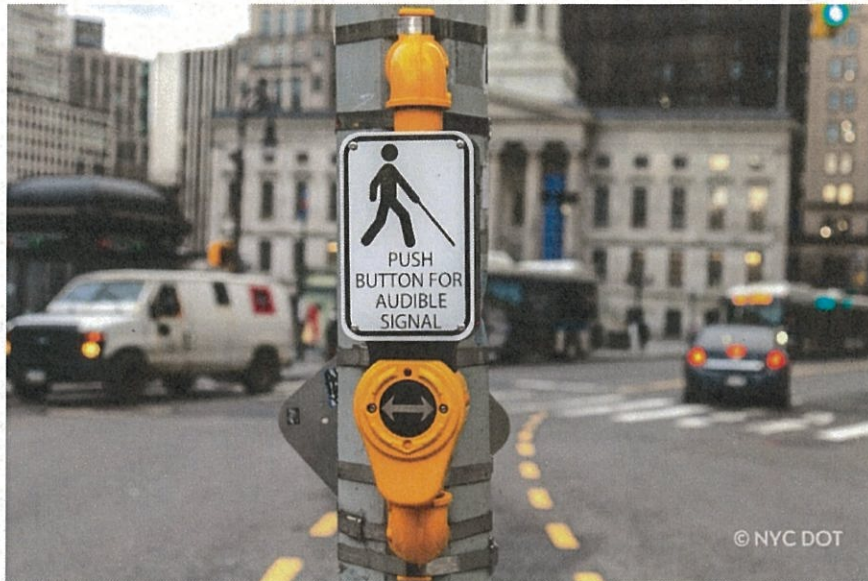
Accessible Pedestrian Signal at Court Street, Brooklyn
