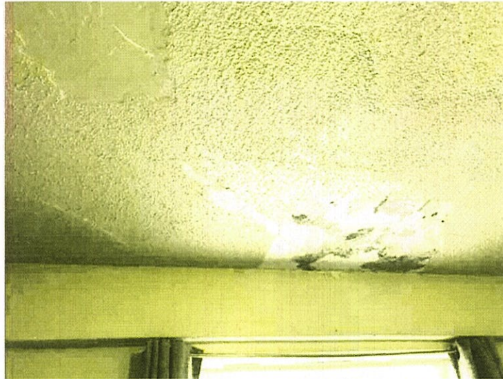
Photo 7: Close up view of a typical slab underside at 17 th floor units showing the localized slab cracking and areas where the moisture infiltration caused the paint peeling off.
