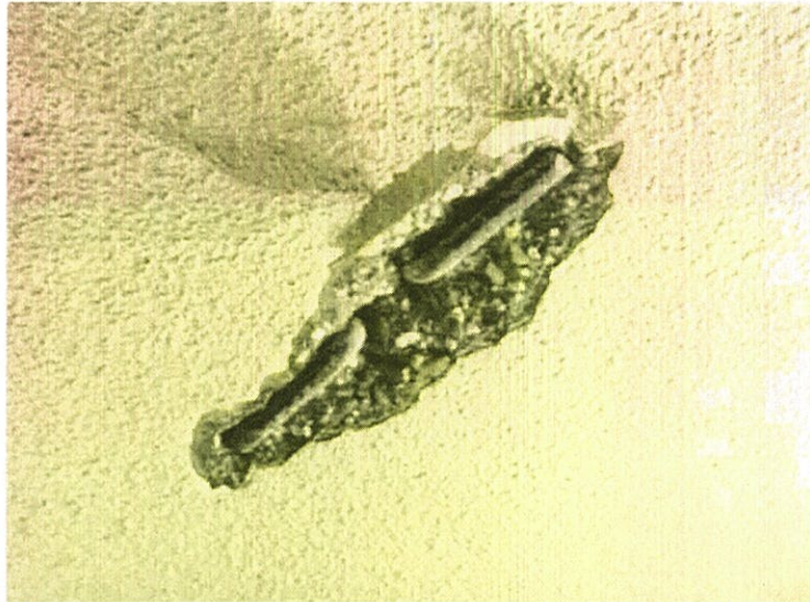
Photo 5: Close up view of a location at 17 th floor underside where the incident occurred on June 30 th .
